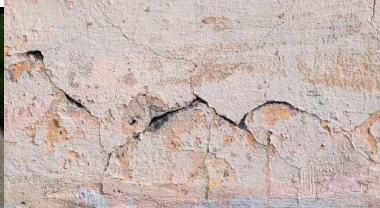
Figure 3.8: Large surface spall
