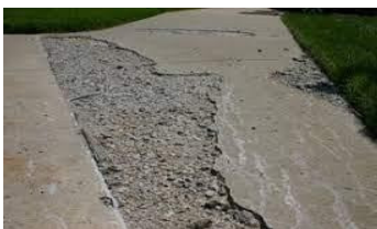
Figure 3.7: Small surface spalls
