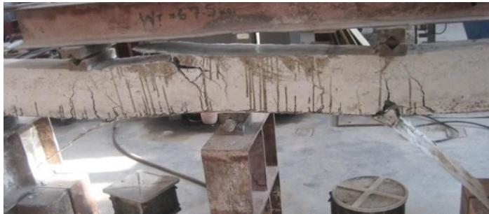
Figure 3.37 FRP sheet separations without concrete
