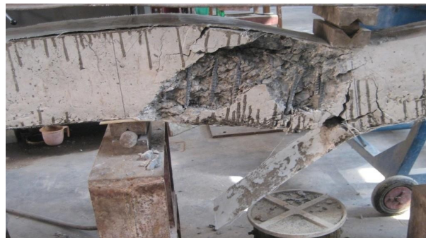
Figure 3.16 Magnified view of the failure of the beam
