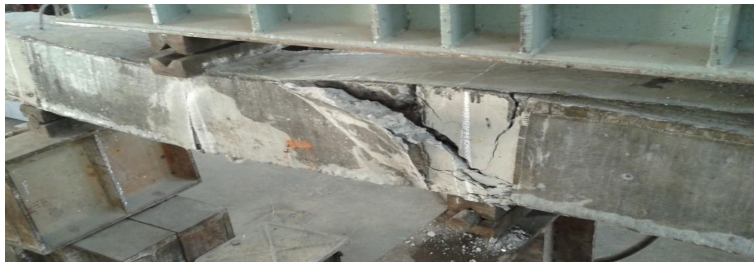
Figure 3.18 Ultimate failure of beam by deboning of FRP with concrete Cover
